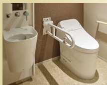
Provision of the sink/ washer fitted with ostomate-friendly toilets
